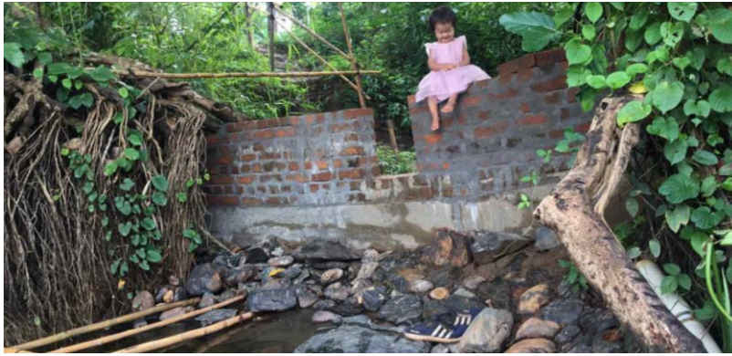
Retaining wall with Ja Ing comfortably sitting and enjoying the river view.
