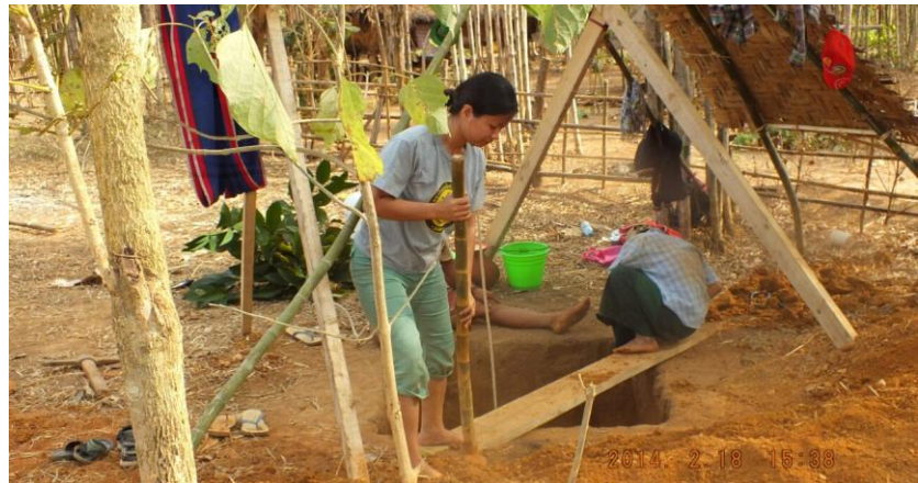
SengPan keeping out any dirt from falling back in after only two days of digging.
